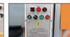
操控箱 Control box.
