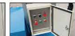
操控箱 Control box.
